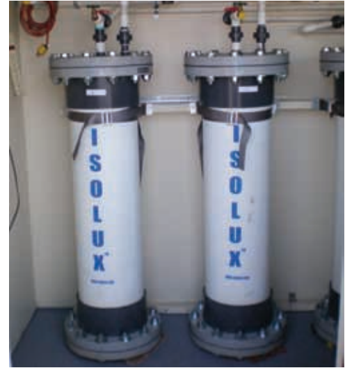
40-GPM system for a church/school complex in California.
