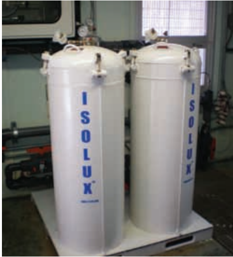
75-GPM module for a community water system site in New Jersey.
