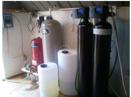
Typical home well water chlorination and pH adjustment system with 80 gallon contact tank.
