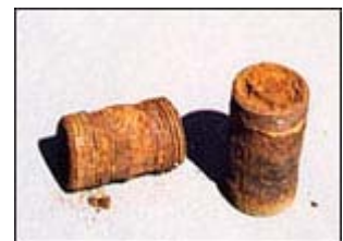
Corroded galvanized pipe nipples from acid water. This water had a pH of 6.2 and required complete replacing of the iron pipes in the home.
