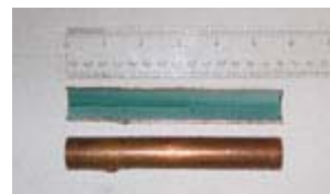
This copper looked fine from the outside. Inside it was being eaten away by the acidic water and eventually sprung pinhole leaks, causing extensive damage to the customers home. We cut away a section of it, above.
