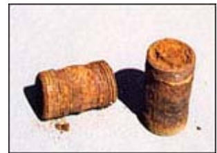
Corroded galvanized pipe nipples from acid water. This water had a pH of 6.2 and required complete replacing of the iron pipes in the home.
